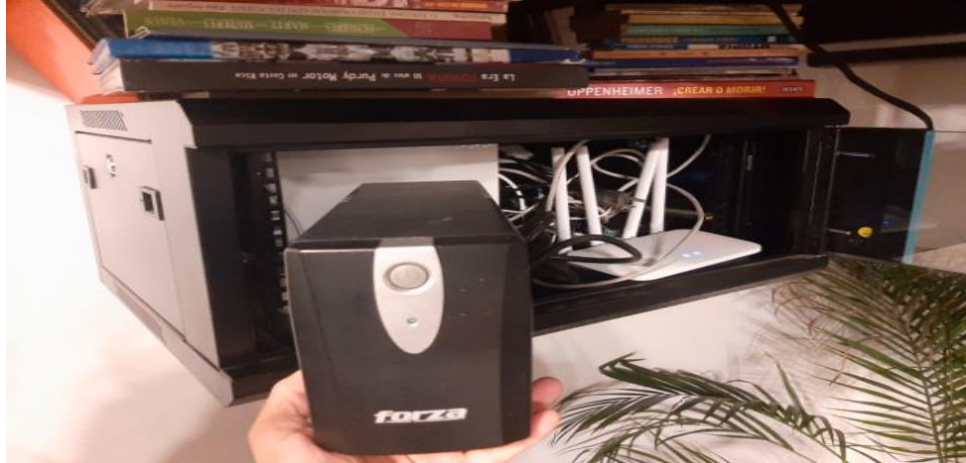
Figura 35 UPS back up.
